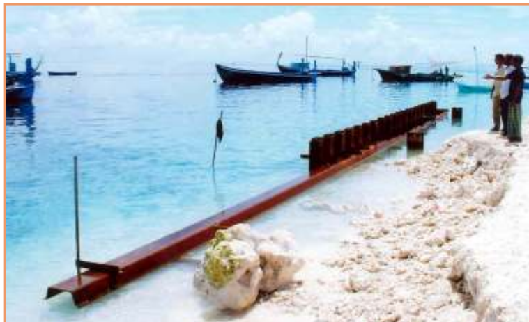
R. Kan'dholhudhoo island land reclamation and eastern harbour sheet-piling underway. The land area had been increased by 45,135.90 sqm.
